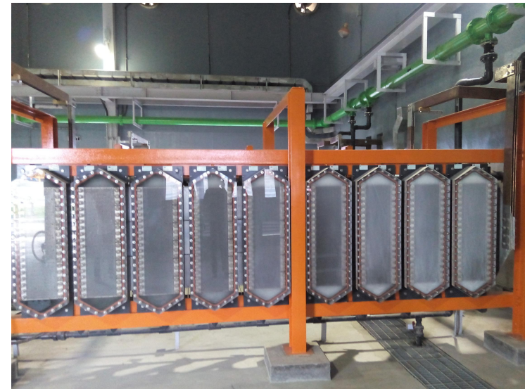
Philippine SLPGC-Calaca CFB Power Plant
