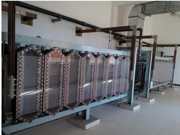
Venezuela Central Power Plant
