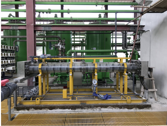
Indonesia Muara Jawa CFSPP Power Plant
